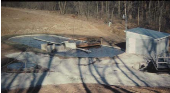
Activated sludge oxidation ditch treatment plant
