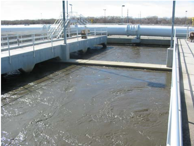
Denitrification Basin Anoxic Stage
