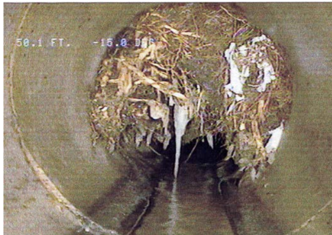
Severe Root Intrusion – Right Grease Buildup - Bottom
