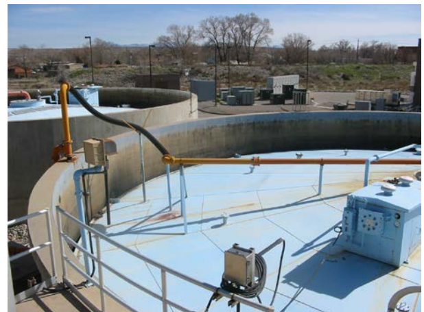
Secondary Digester with Floating Cover
