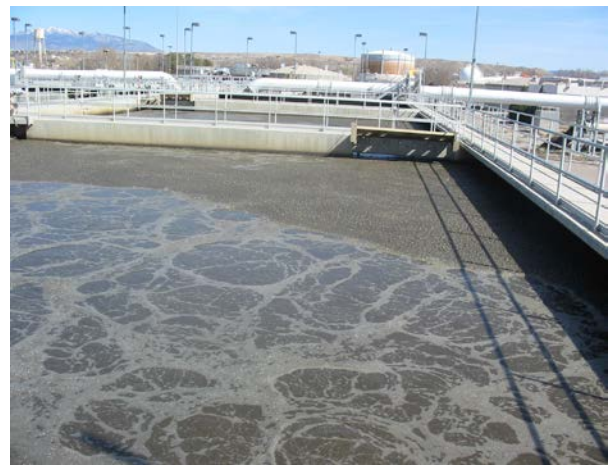
Denitrification Basin Final Aeration Stage
