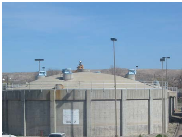
Primary digester with mechanical mixers
