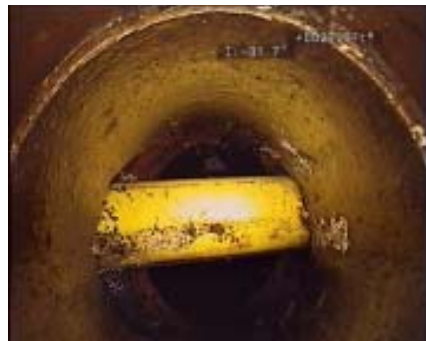
Sewer pipe pierced by a gas delivery line.
